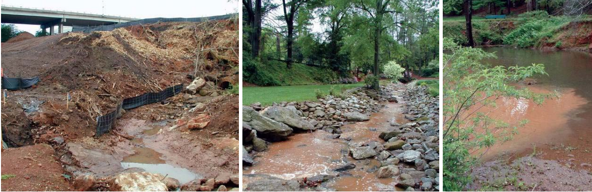
This development site in Greenville is typical of many in the region, with extensive bare dirt and failing erosion control structures. It took only a 20-minute shower to send a plume of sediment down to the nearest stream and into the Reedy River.
