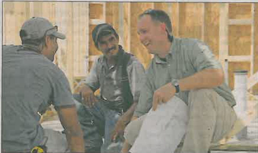
Todd Usher, president of Addison Homes, visits a job site where one of the company's homes is being built.
