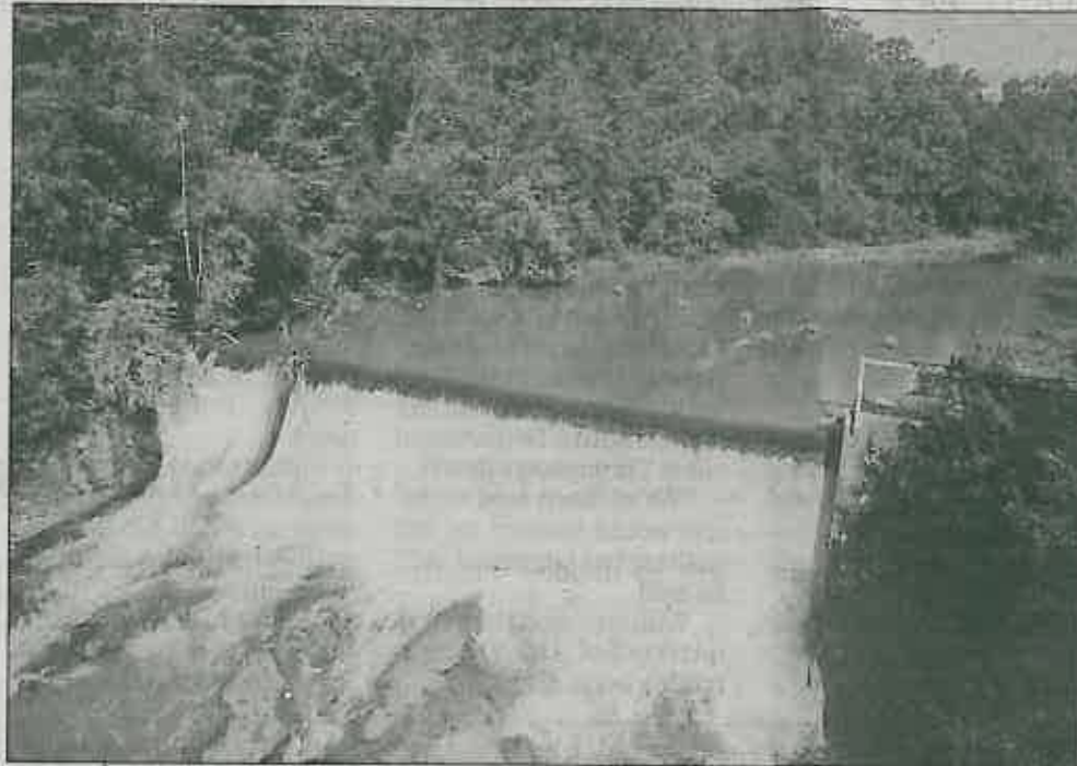
The dam on Twelve Mile Creek at the Catechee Mill site is one of two that will be destroyed to counter PCB contamination in the creek and Hartwell Lake.
