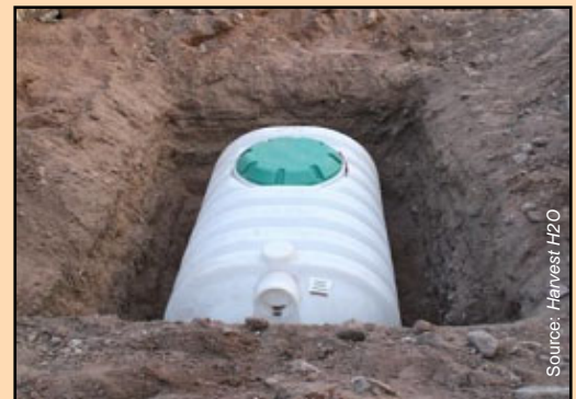
In-ground polyethylene cistern
